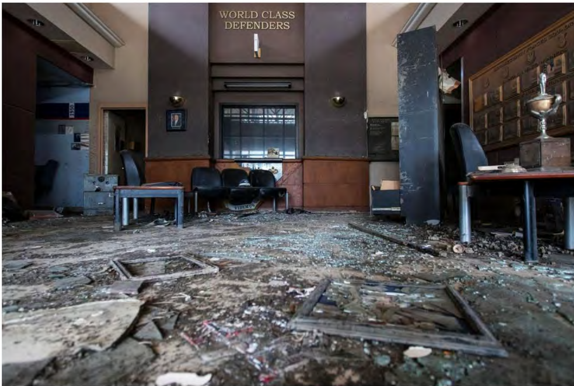
Shattered glass and other debris litters the entryway of the 55th Security Forces Squadron headquarters building six months after it was damaged in the March 2019 floods.
