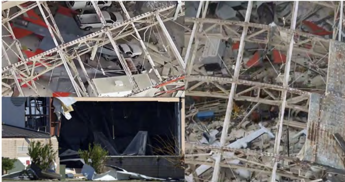
Hurricane Michael hit U.S.A.F Tyndall: Two F-16 & two F-22 can be spotted in a roofless hangar
