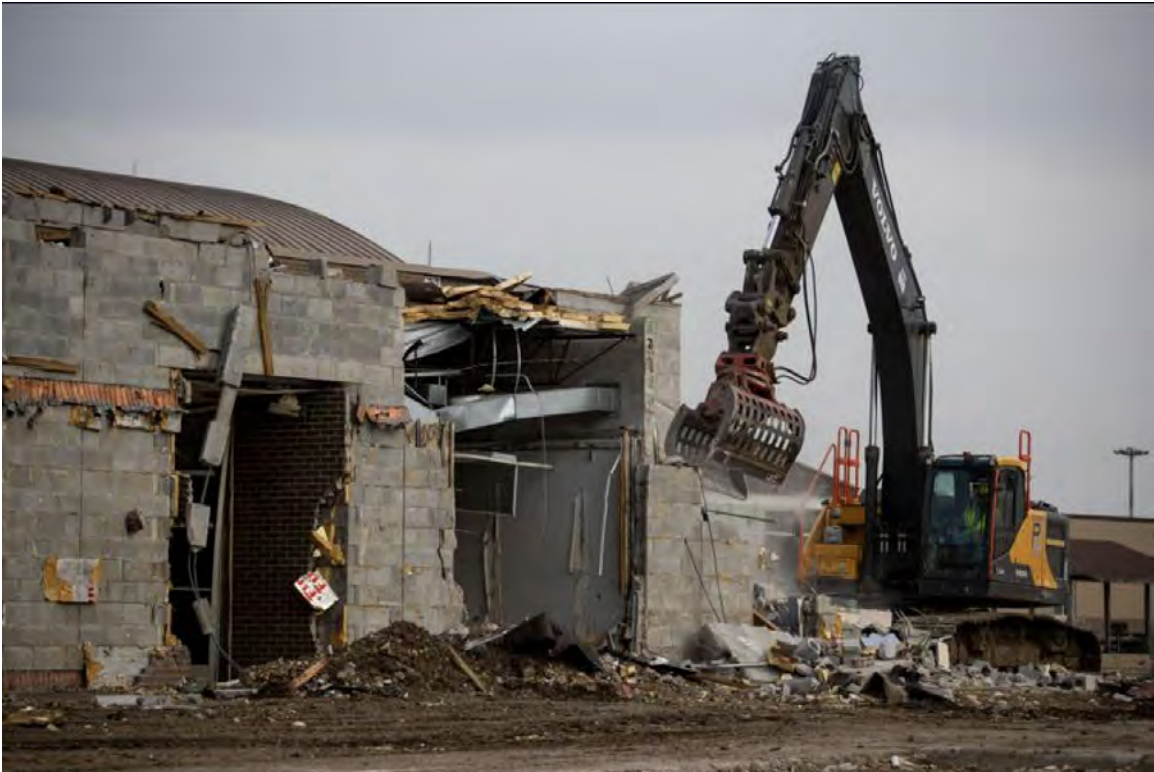
Figure 20. Demolition Started Three Years After the 2019 Flood. Sixty buildings were damaged beyond repair and will be demolished in phases. Image accessed from: https://omaha.com/news/local/offutt-offers-update-on-rebuilding-efforts-following-catastrophic-2019-flooding/article_ca633c86-a549-11ec-a01a-5b6e50743343.html
