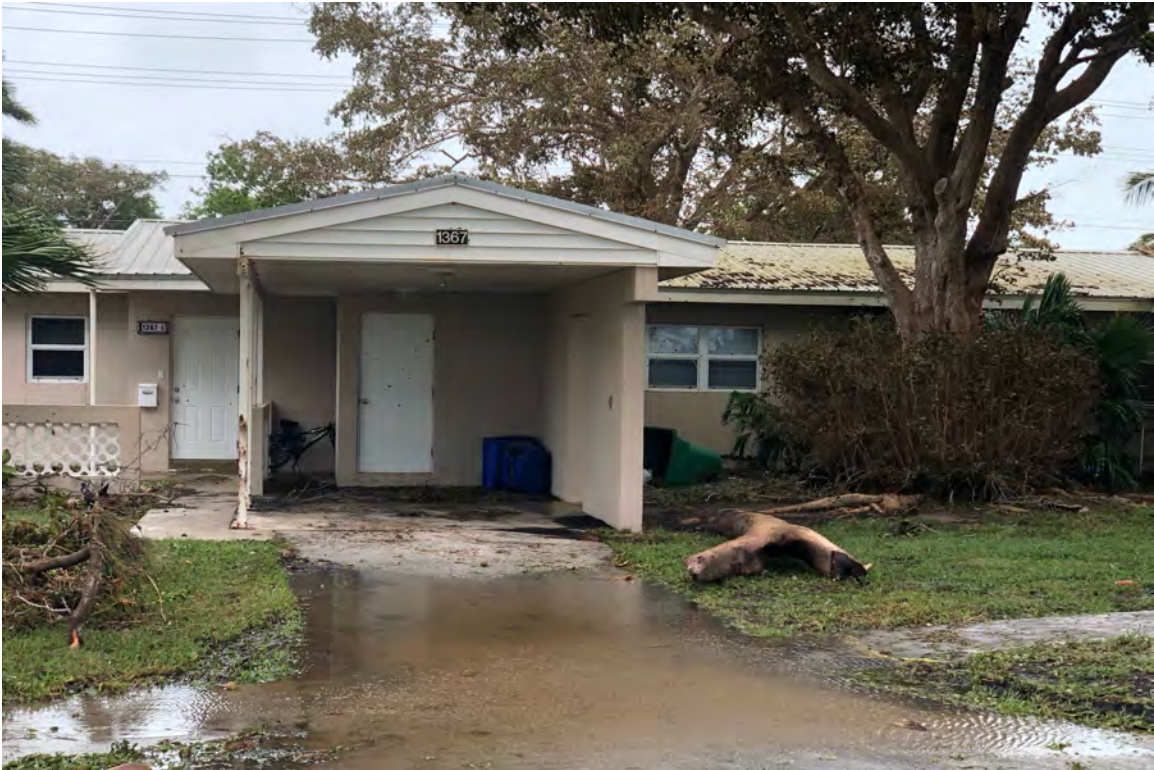
Figure 33. Debris from Hurricane Ian and Damage to NAS Key West Base Housing. In addition to widespread flooding, the military housing units at NAS Key West were damaged by debris that became airborne during Hurricane Ian. Image accessed from: https://www.defense.gov/News/Releases/Release/Article/3173718/naval-air-station-key-west-evacuates-impacted-base-housing-due-to-hurricane-ian/
