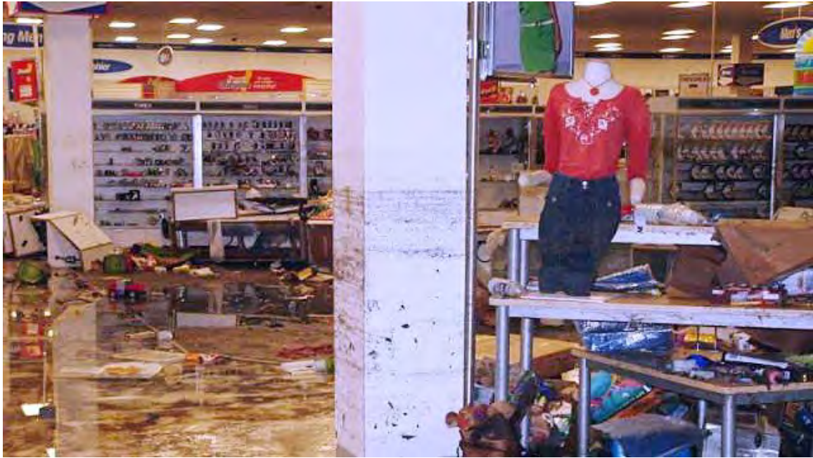
Figure 4. Shopping Center Damage from Hurricane Katrina. Hurricane Katrina caused extensive flooding at Keesler AFB, including the military support and shopping privilege center. As seen here, floodwaters submerged halfway up the support column in the clothing store. Image accessed from: https://publicaffairs-sme.com/FamilyServingFamily/2021/09/03/flashbackfriday-the-keesler-exchanges-resiliency-after-hurricane-katrina/
