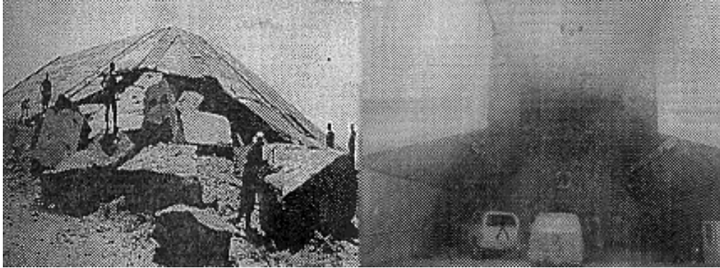
Figure 1. Exterior (left) and interior (right) photographs of an aircraft shelter hit by two bombs in the Gulf War (Cohen [6]). Apparently heavy damage is actually not.
